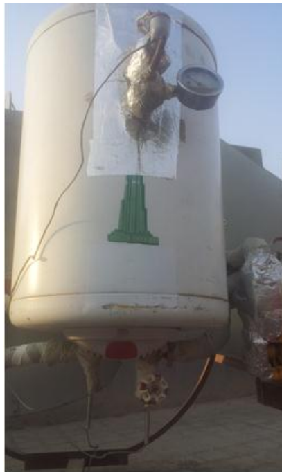
Plate (4.4): Storage Tank
