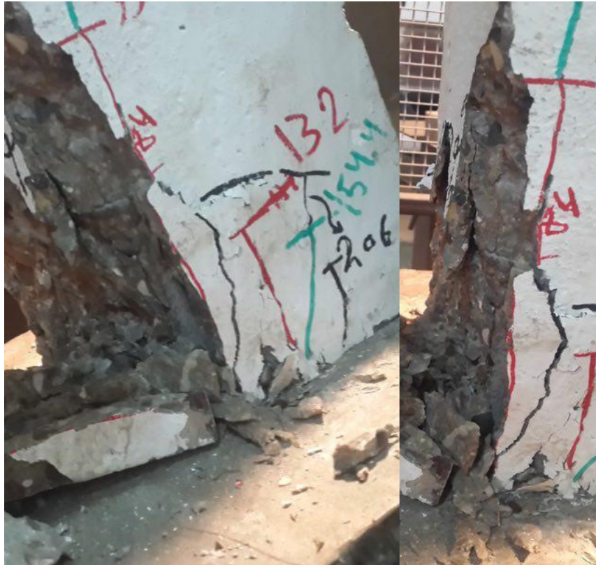
Plate (4-25): Failure Pattern for Column (HS2)
