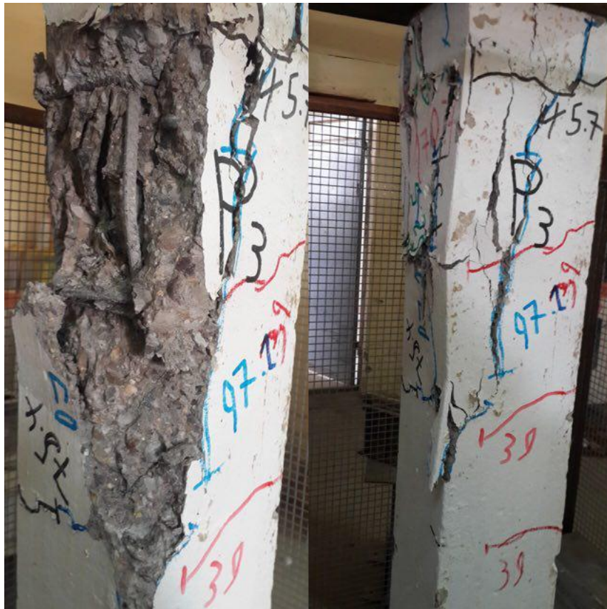
Plate (4-9): Failure Pattern for column (P3)
