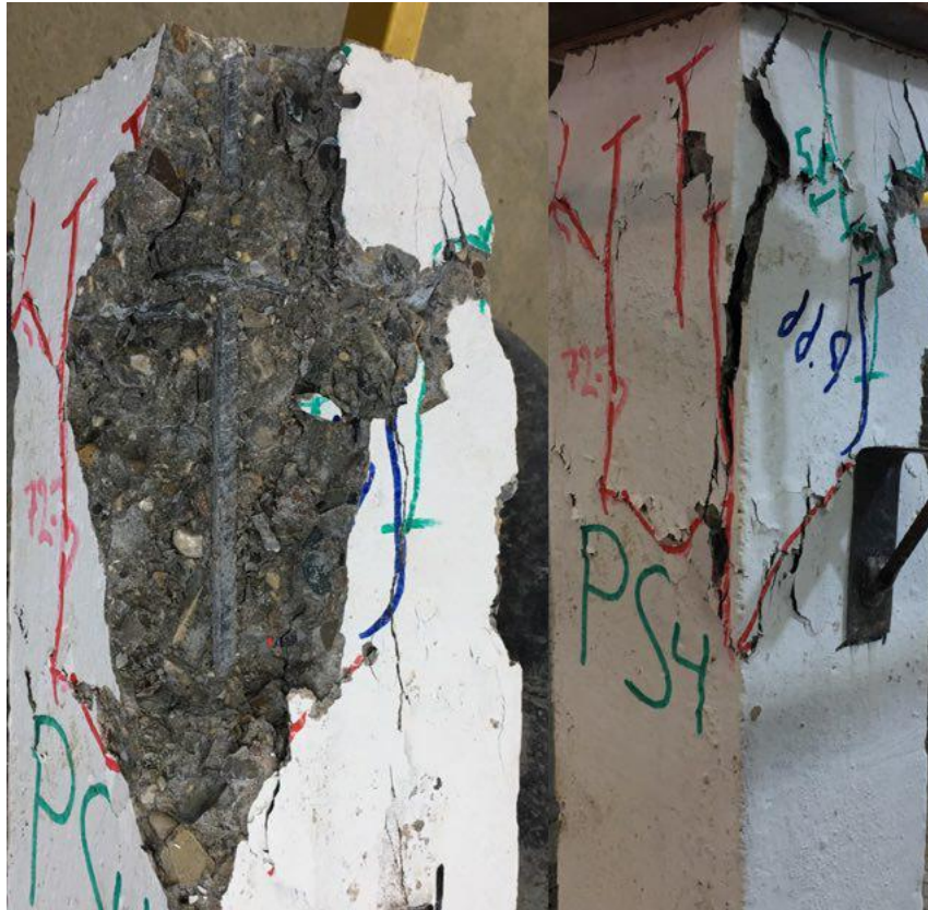
Plate (4-23): Failure Pattern for Column (PS4)
