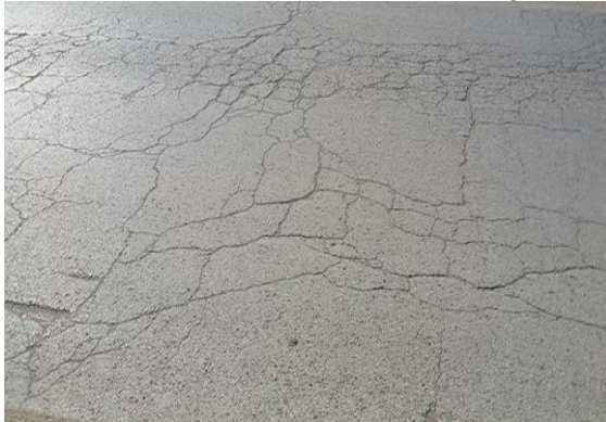
C. Alligator or Fatigue Cracking
