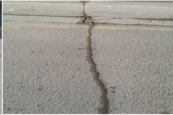
B. Transfer Cracking
