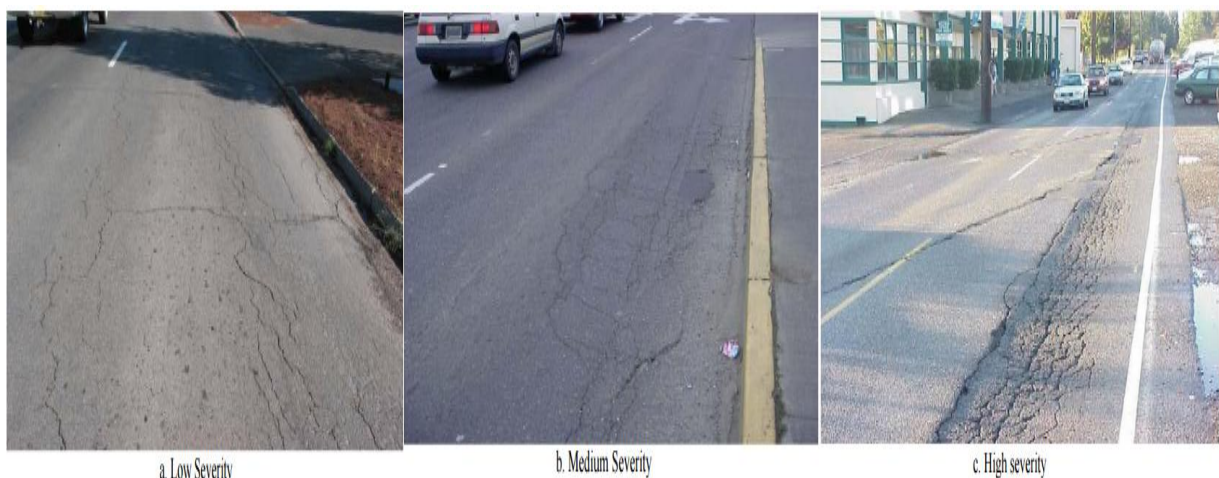
Figure (A-1) Alligator Cracking
