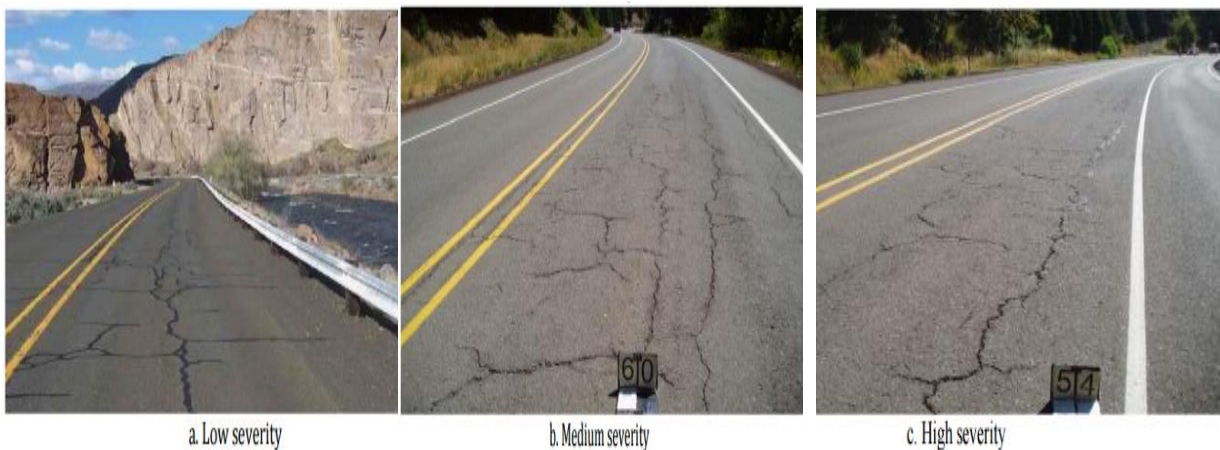
Figure (A-3) Block cracking
