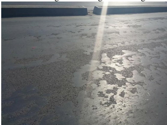
E. Bleeding and Raveling
