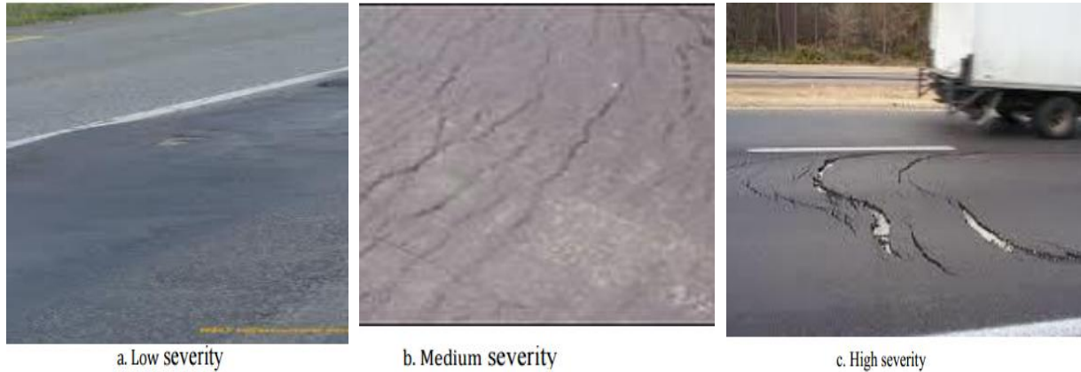
Figure (A-4) Slippage cracking
