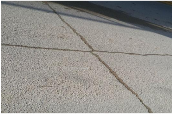
A. Joint Reflection Cracking
