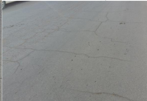
D. Block Cracking
