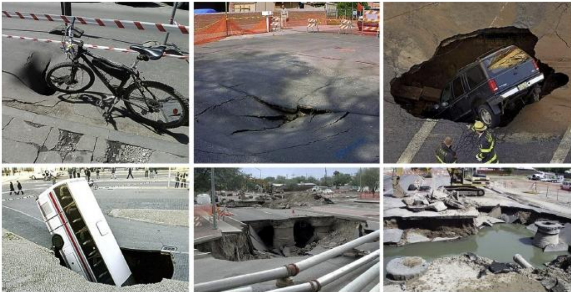
Figure (2-16) road consequences by pipe defects(Kuliczowska, 2016)
