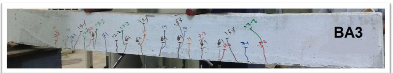
Figure (4-66): Crack patterns of beam BA3
