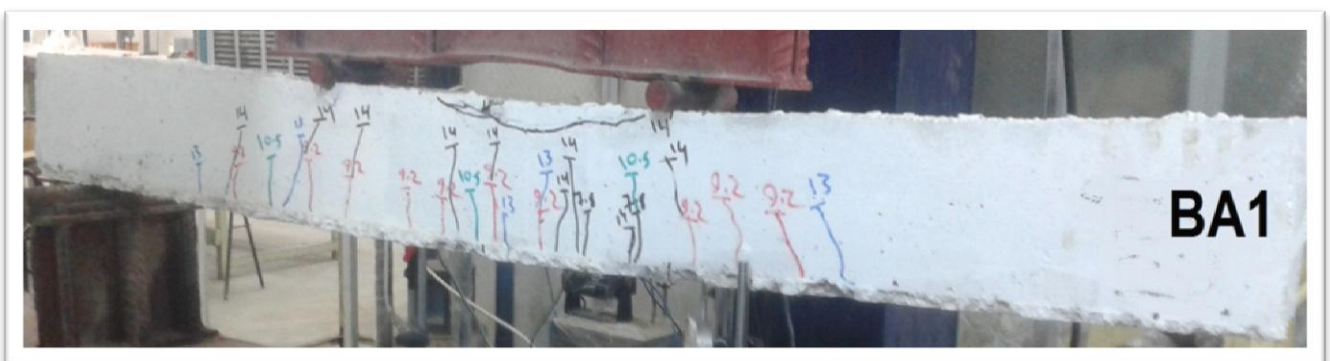
Figure (4-55): Crack patterns of beam BA1
