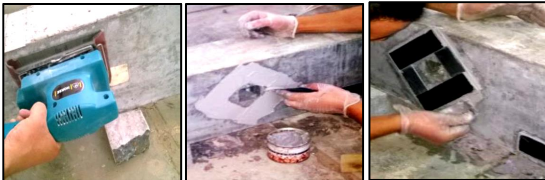
Plate 2. 7: Strengthening by CFRP at the Web Opening for Beams Tested by Abtan and AbdulJabbar, (2019)
