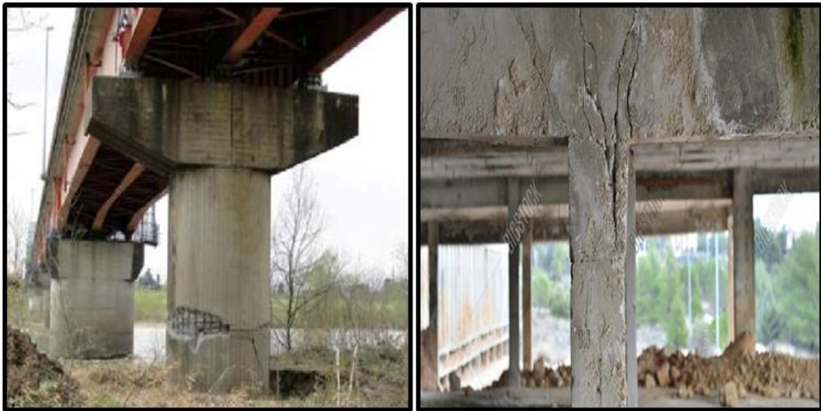
Fig 1.1 Samples of damaged columns caused by earthquakes
