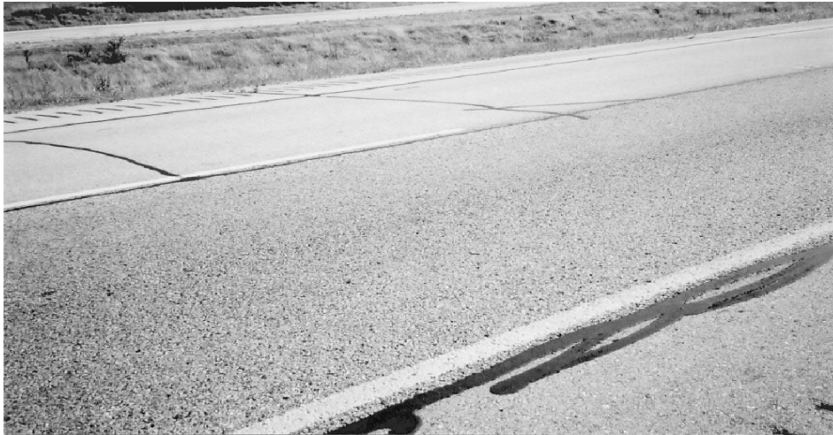
Plate 2- 6 Reduced reflective cracking in SMA (right lane) versus conventional mix (left lane) (Watson, 2003).
