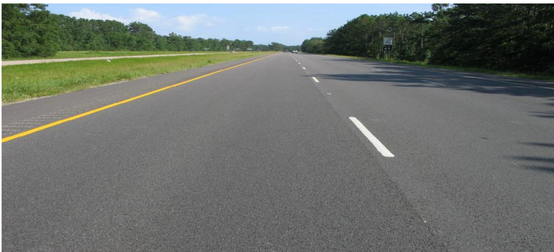
Plate 2- 7 Reduced reflective cracking in SMA (right lane) versus conventional mix (left lane) (Watson, 2003).
