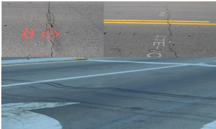
Plate 2- 14 Minor Distresses of Pavement Surface (Chen et al., 2015, NAPA, 2002)
