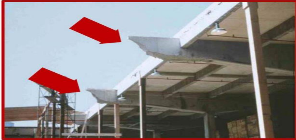
Plate 1-2: Shear Failure of Air Force Warehouse Beams ( Collins et al. 2008 )
