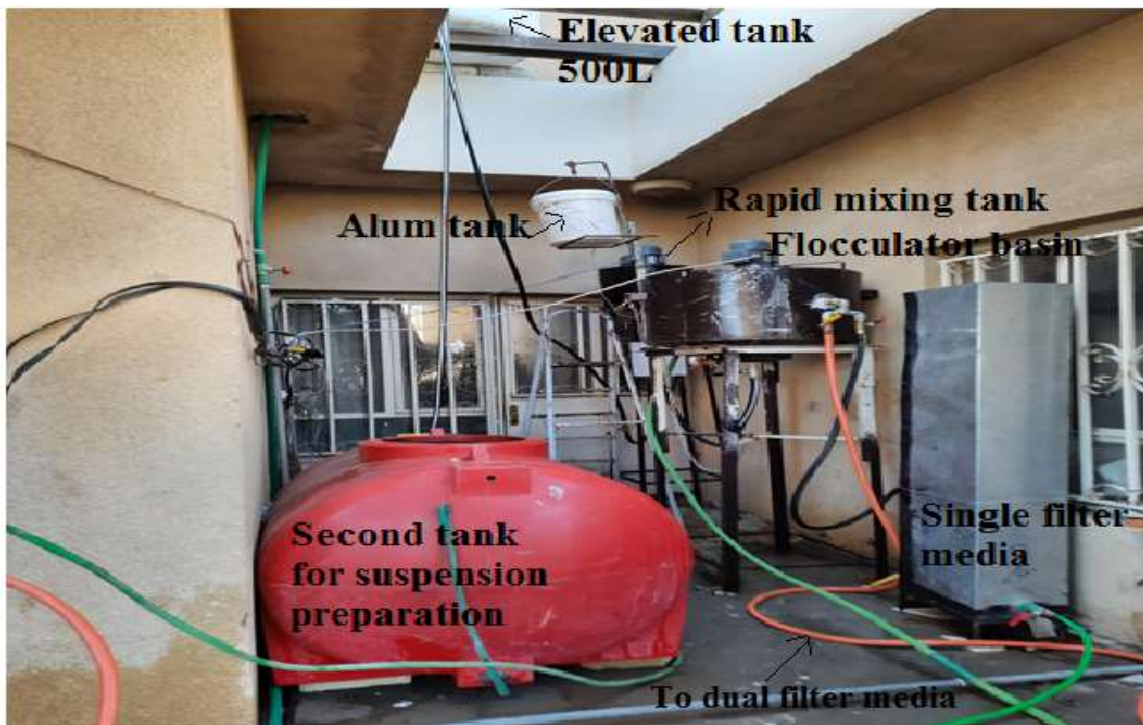
Plate:(3-2) Ground level tank, Elevated tank ,Rapid mixing tank, Clariflocculator tank and Single filter media arrangement in the pilot plant .
