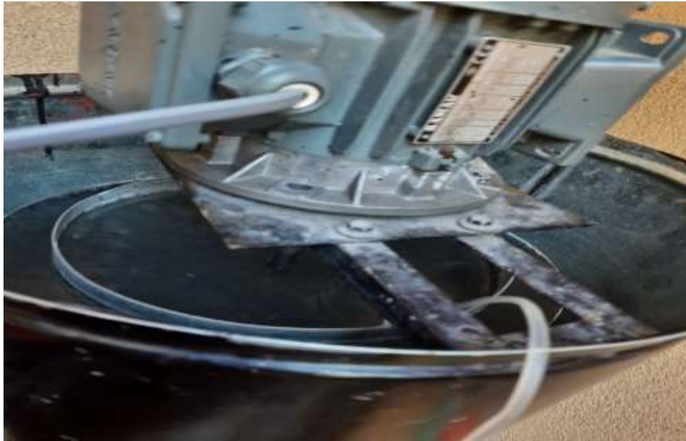
Plate (3-4): Flash mixer tank.
