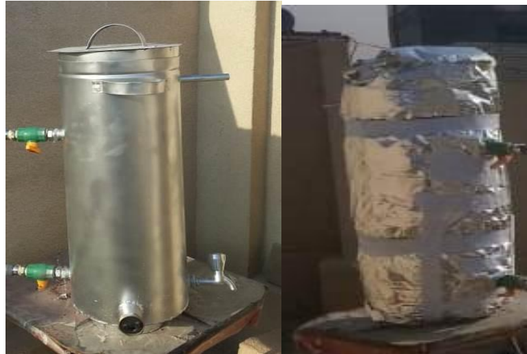
Figure 4-3. Water tank used in the solar heating system
