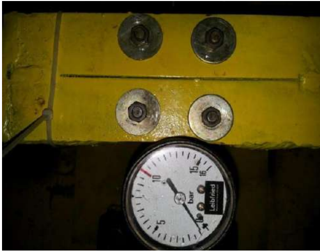
Figure (4-13) Pressure gauge
