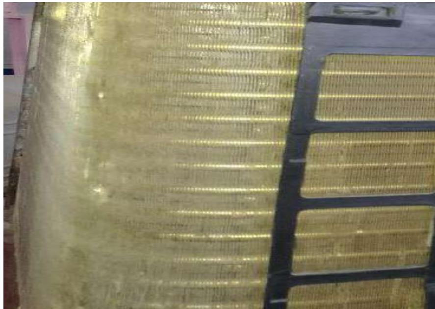
Figure (4.3): The condenser.
