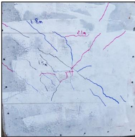
H.S 70 mm Crack patterns
