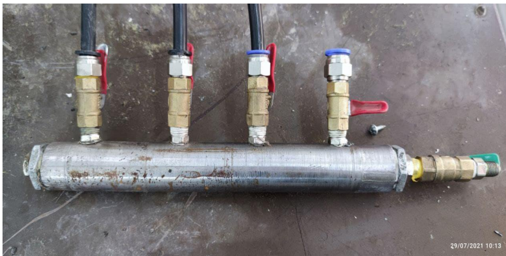
Figure (4.22): Vacuum system manifold
