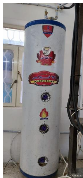
Figure (4.18): Hot water tank (electric boiler) utilised in the test facility
