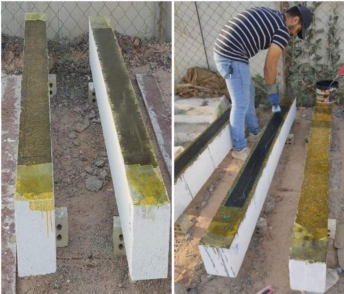
b) Apply a layer of epoxy primer c) Laying epoxy adhesive and applying CFRP
