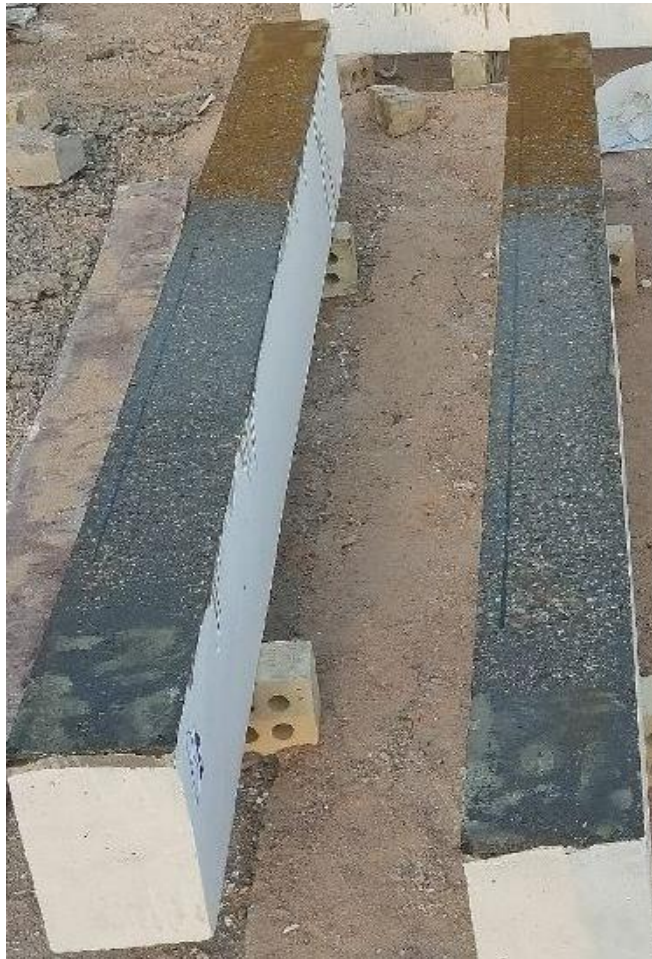
a) Skim the bottom surface and wash it in preparation for the epoxy primer
