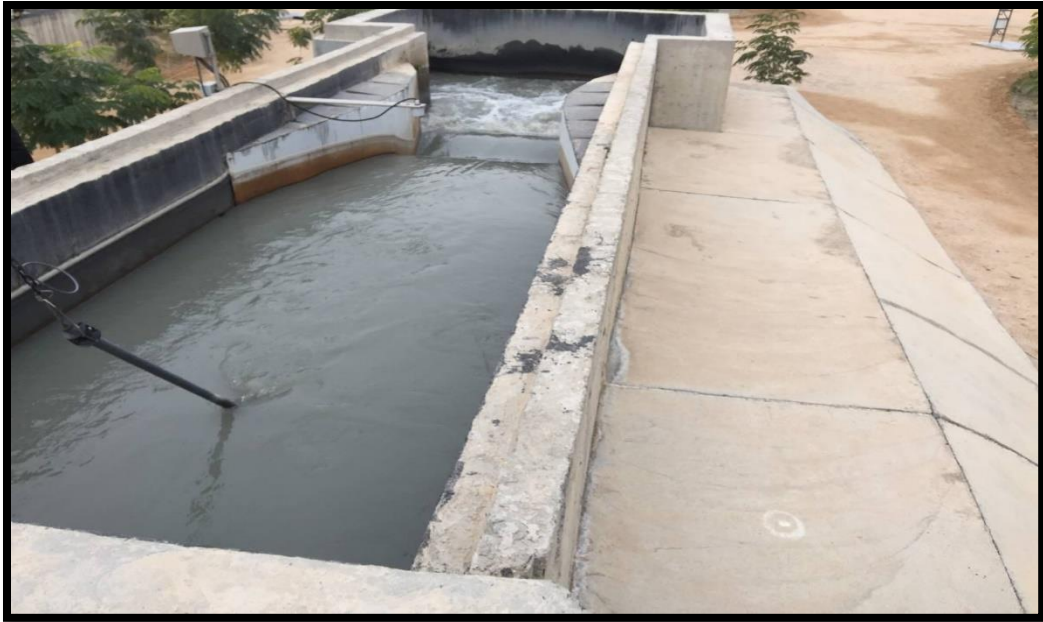
Figure 3-6: Parshall flume unit in Karbala WWTP.
