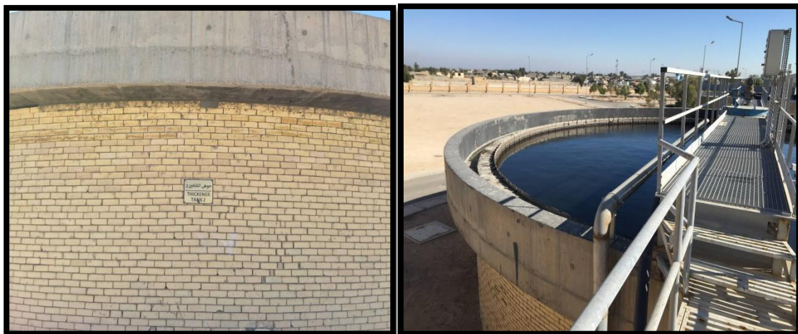
Figure 3-11: gravity thickener basin in Karbala WWTP.
