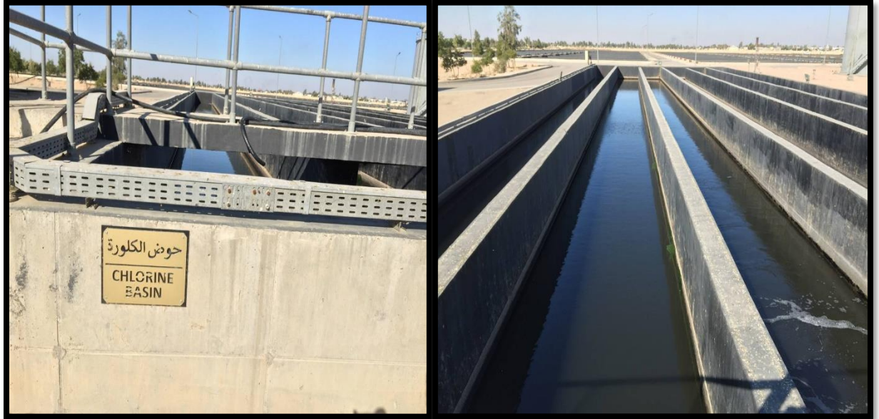
Figure 3-10: Chlorination basin in Karbala WWTP.
