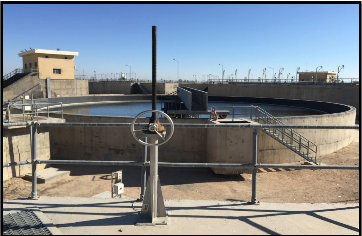
Figure 3-7: Primary sedimentation tank in Karbala WWTP.
