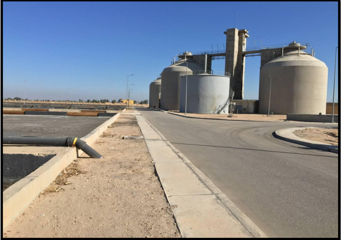
Figure 3-15: Biogas treatment reactor in Karbala WWTP.
