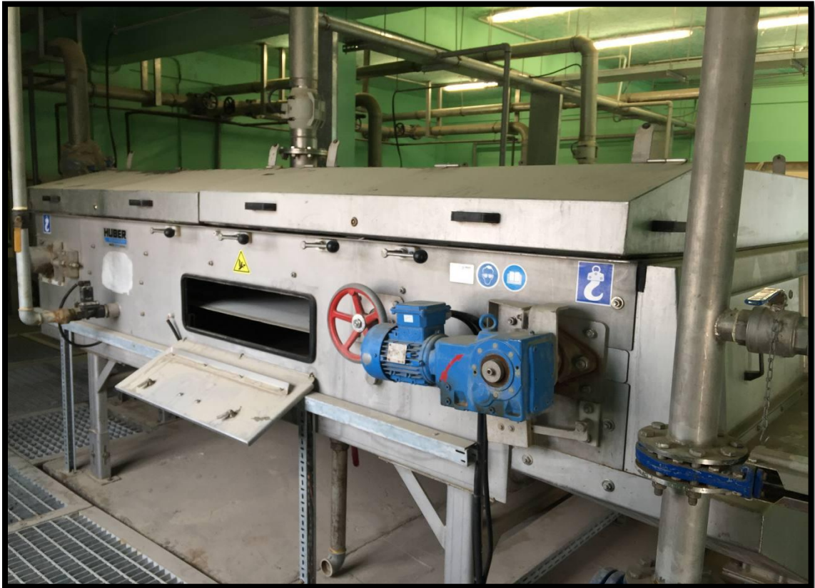
Figure 3-12: Mechanical thickener units in Karbala WWTP.
