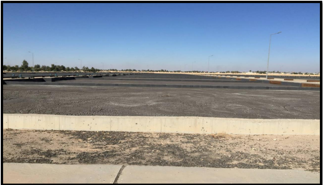
Figure 3-14: drying bed in Karbala WWTP.
