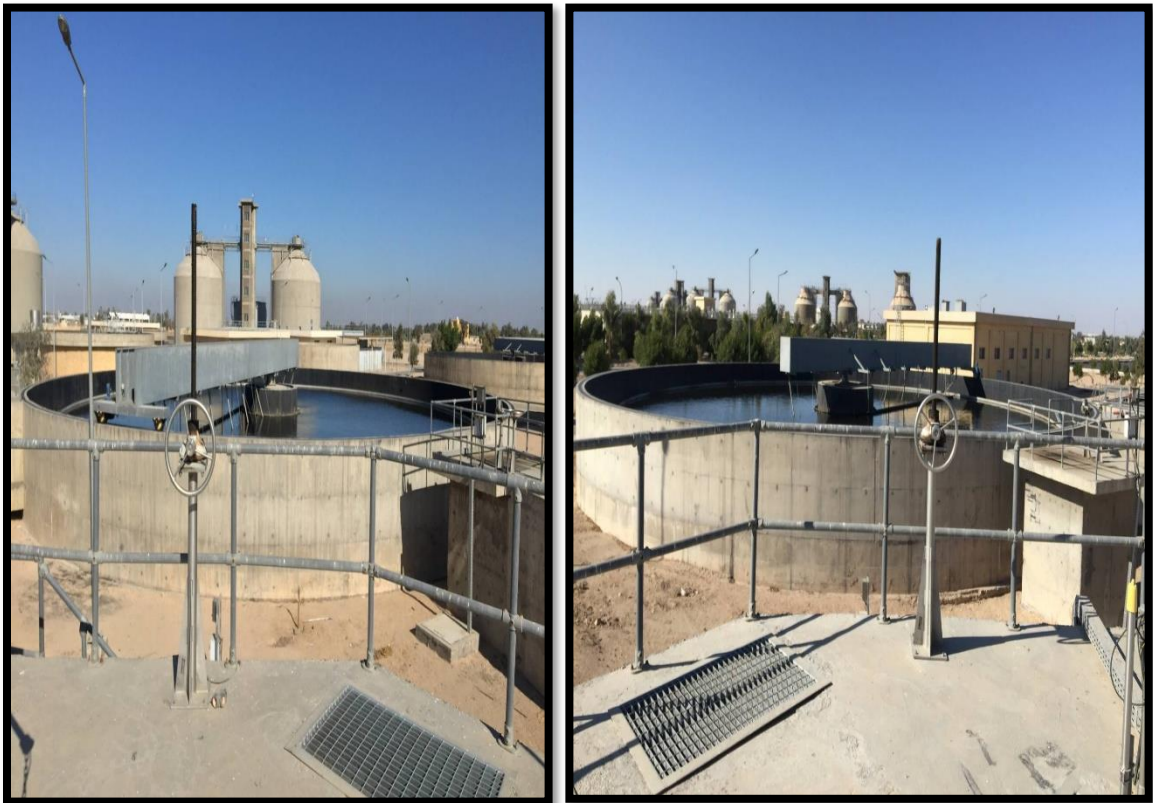
Figure 3-9: Secondary clarifier tank in Karbala WWTP.
