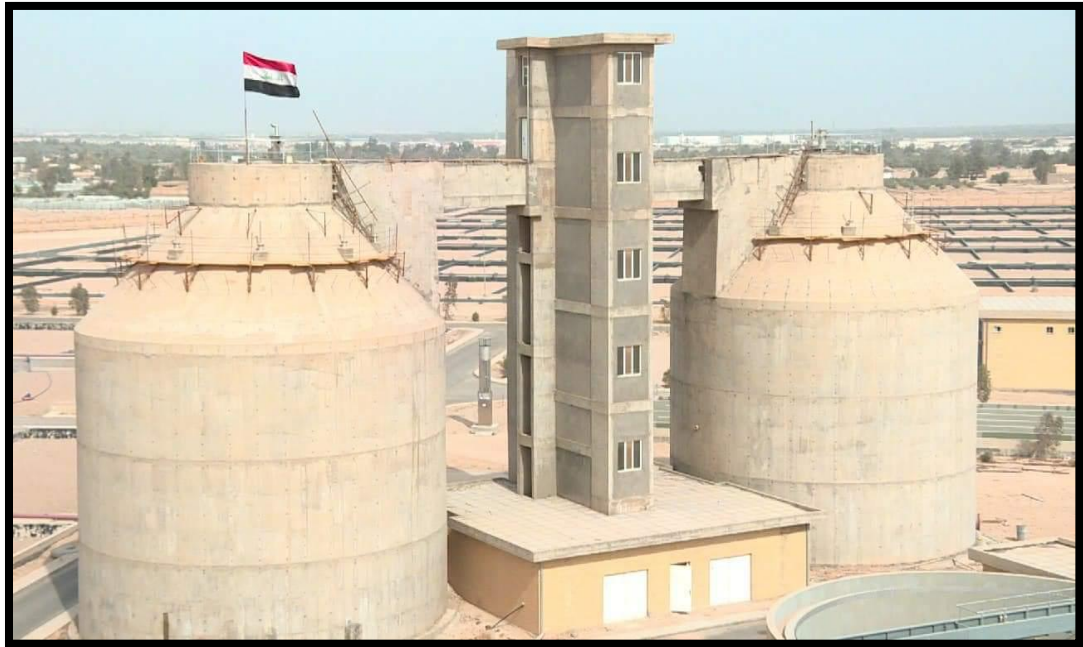
Figure 3-13: Anaerobic digester in Karbala WWTP.
