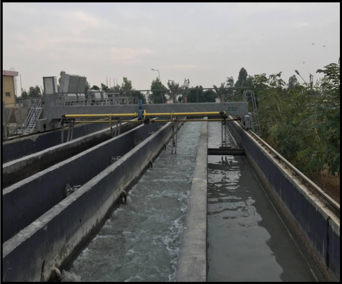
Figure 3-5:Grit chamber in Karbala WWTP.
