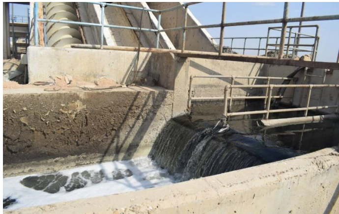
Figure 3-8. Open channel in the WWTP of AL-Samawah taken by Zahraa on October 28 th , 2021).
