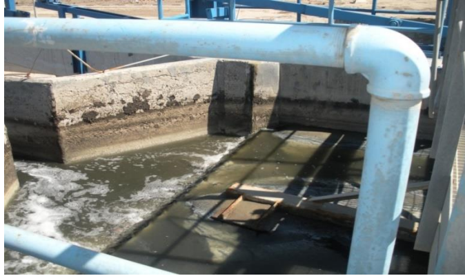
Figure 3-5. Grit Basins in AL-Samawah WWTP
