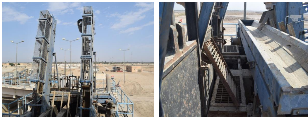
Figure 3-4. Screens in WWTP of AL-Samawah (taken by Zahraa on October 28 th , 2021).
