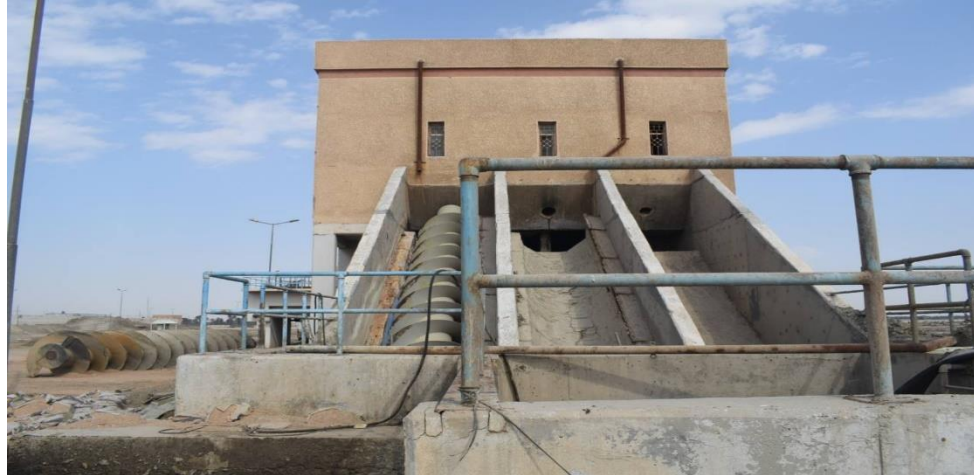
Figure 3-3. Screw Pump in the Inlet of Flow to AL-Samawah WWTP taken by Zahraa on October 28 th , 2021).
