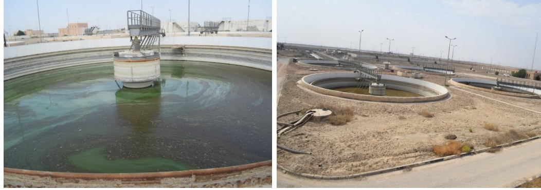
(a) (b) Figure 3-7. Secondary Clarifier Basins in WWTP of AL-Samawah taken by Zahraa on October 28 th , 2021).
