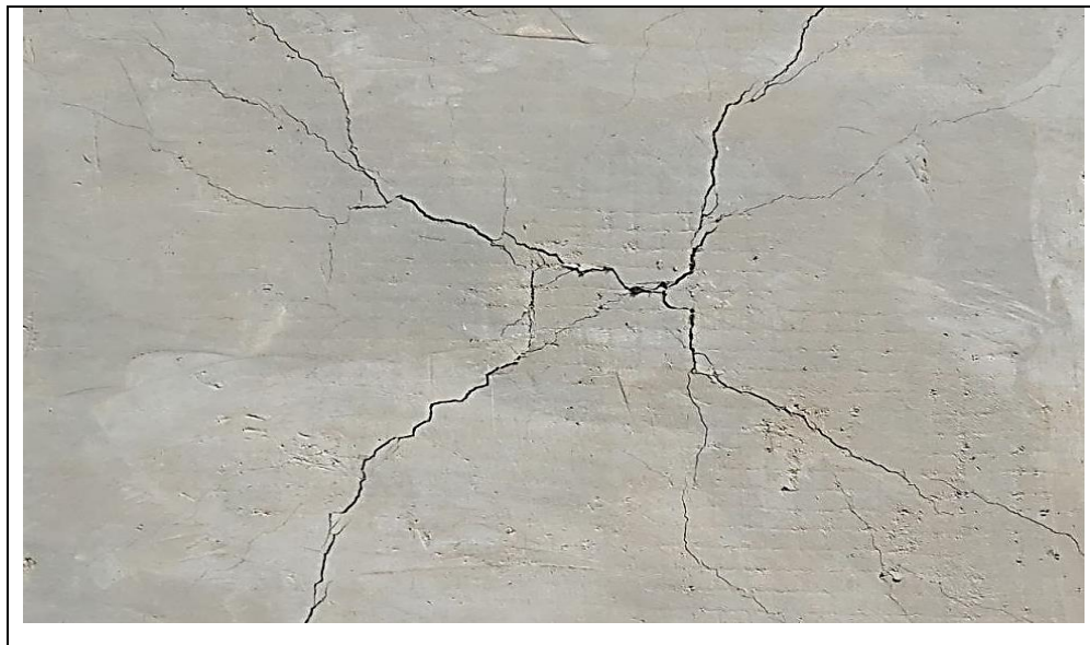
Figure 4-9: Details of flexural cracks in the mortar of the TRM composites (S5).
