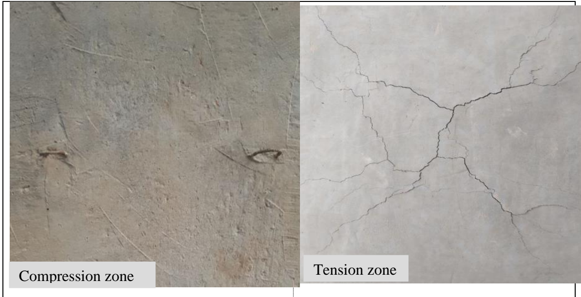
Figure 4-12: Rupture of the carbon textile and formation of flexural cracks in the mortar of the TRM composites (S9).
