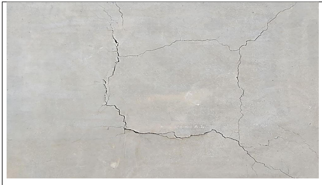
Figure 4-11: Details of flexural cracks in the mortar of the TRM composites (S6).
