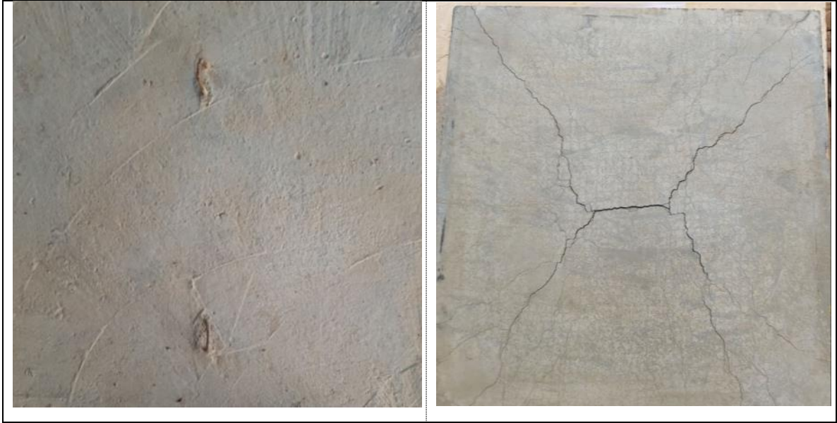
Figure 4-14: Rupture of the carbon textile and formation of flexural cracks in the mortar of the TRM composites (S10).
