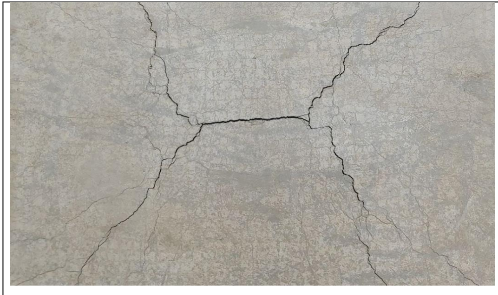
Figure 4-15: Details of flexural cracks in the mortar of the TRM composites (S10).
