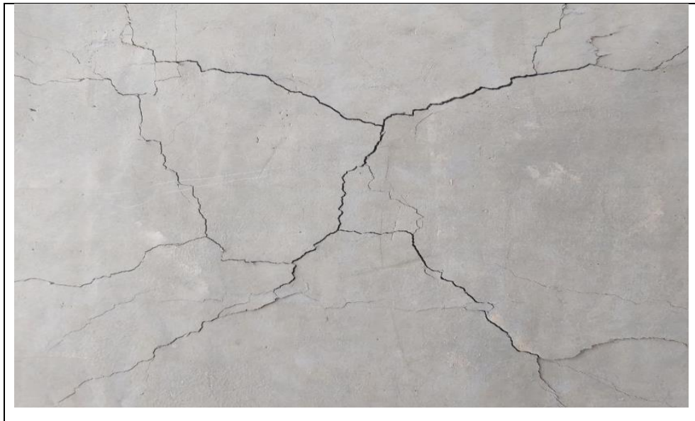
Figure 4-13: Details of flexural cracks in the mortar of the TRM composites (S9).
