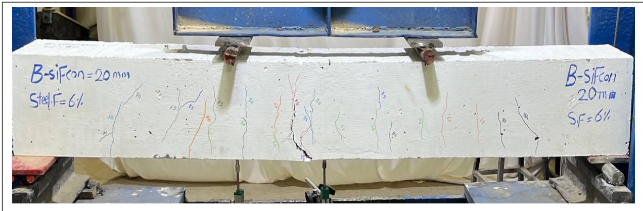
Figure 4.8: Cracking Pattern of Specimen B20-6.
