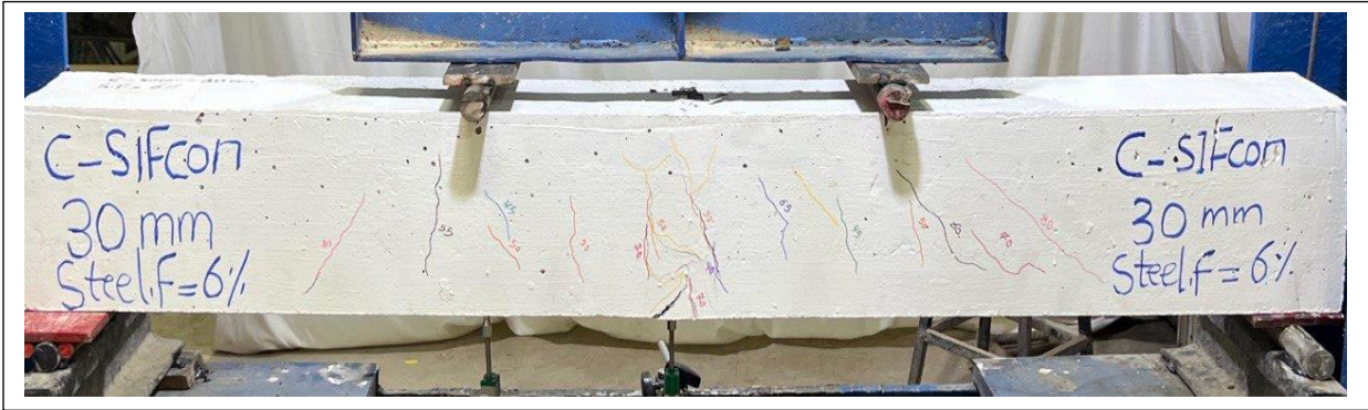
Figure 4.11: Cracking Pattern of Specimen C30-6.
