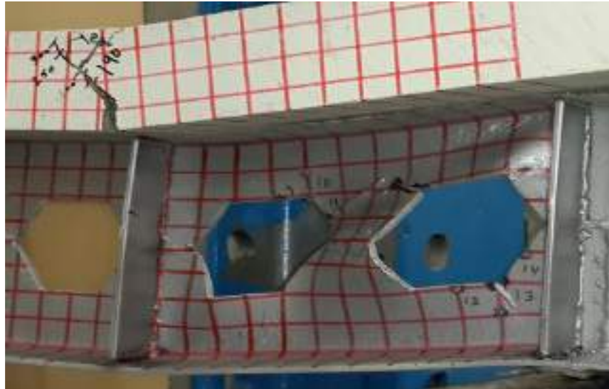
Plate 1-2: Shear Buckling in the Web Post of Castellated Beam [3].
