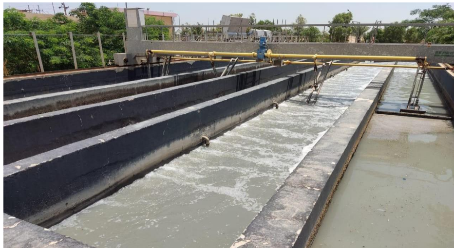
Figure 3-3. Grit chamber of Karbala WWTP.
