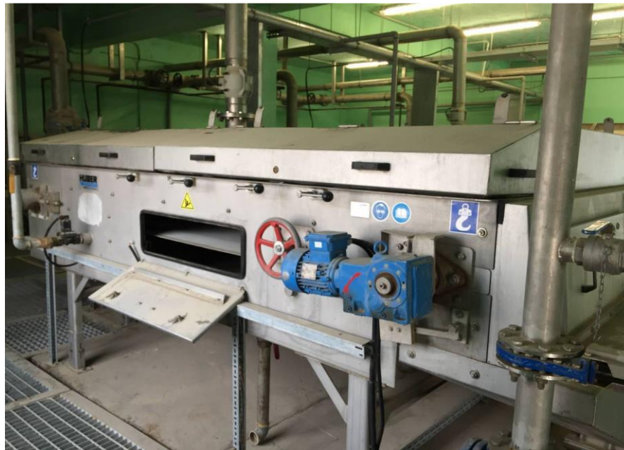
Figure 3-9. Mechanical thickener units in Karbala WWTP.
