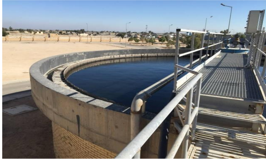
Figure 3-8. Gravity thickener basins of Karbala WWTP.
