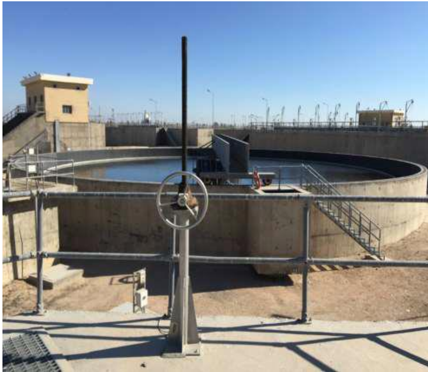
Figure 3-5. Preliminary sedimentation tank of Karbala WWTP.
