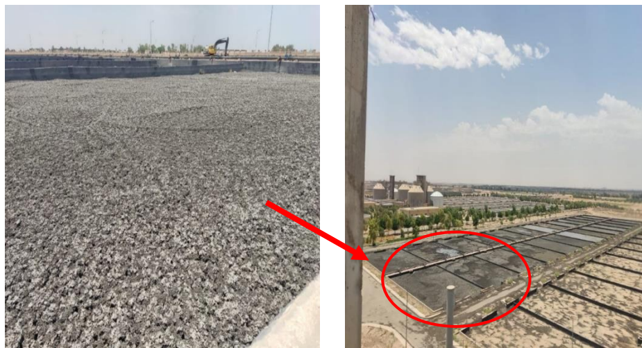
Figure 3-11. Drying bed of Karbala WWTP.
