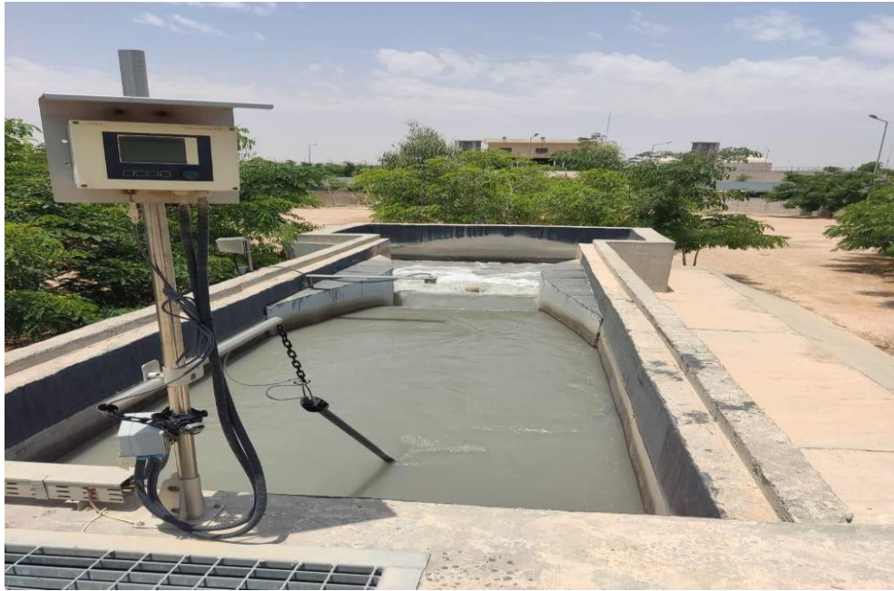
Figure 3-4. Parshall flume unit of Karbala WWTP.
