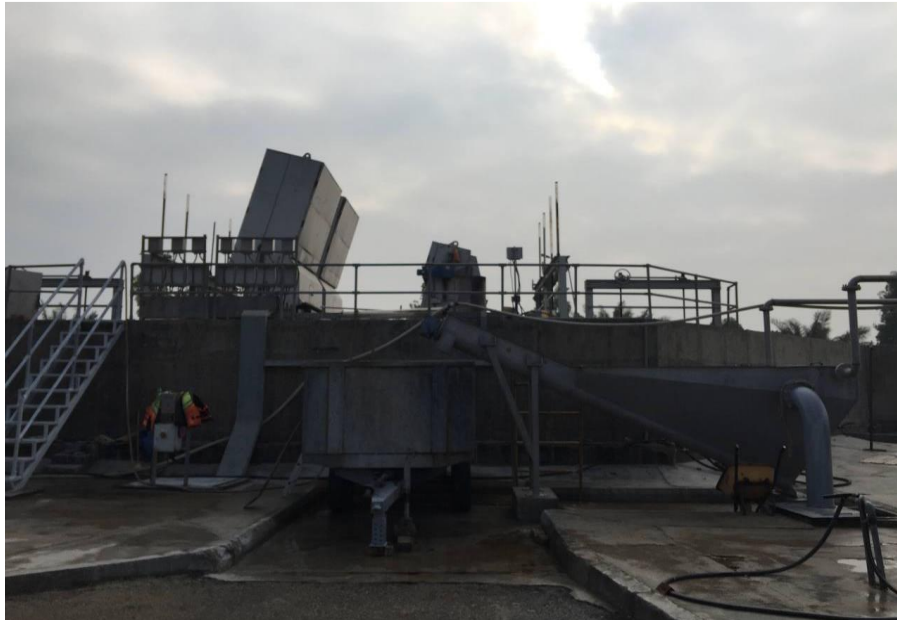
Figure 3-2. Course and fine screen units in Karbala WWTP.
