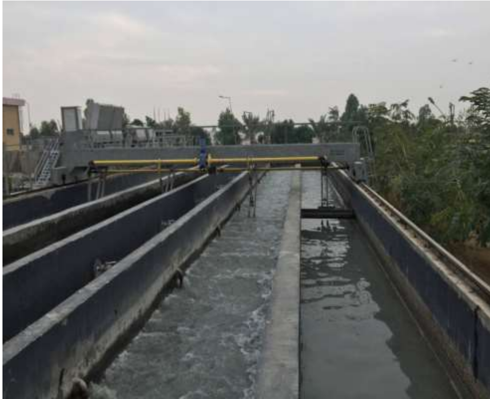
Figure 3-3: Grit Chamber of Karbala WWTP
