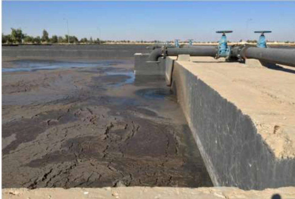
Figure 3-8: Drying Bed in Karbala WWTP
