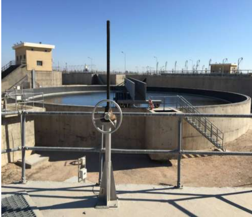
Figure 3-5: The Primary Sedimentation Tanks of Karbala WWTP .
