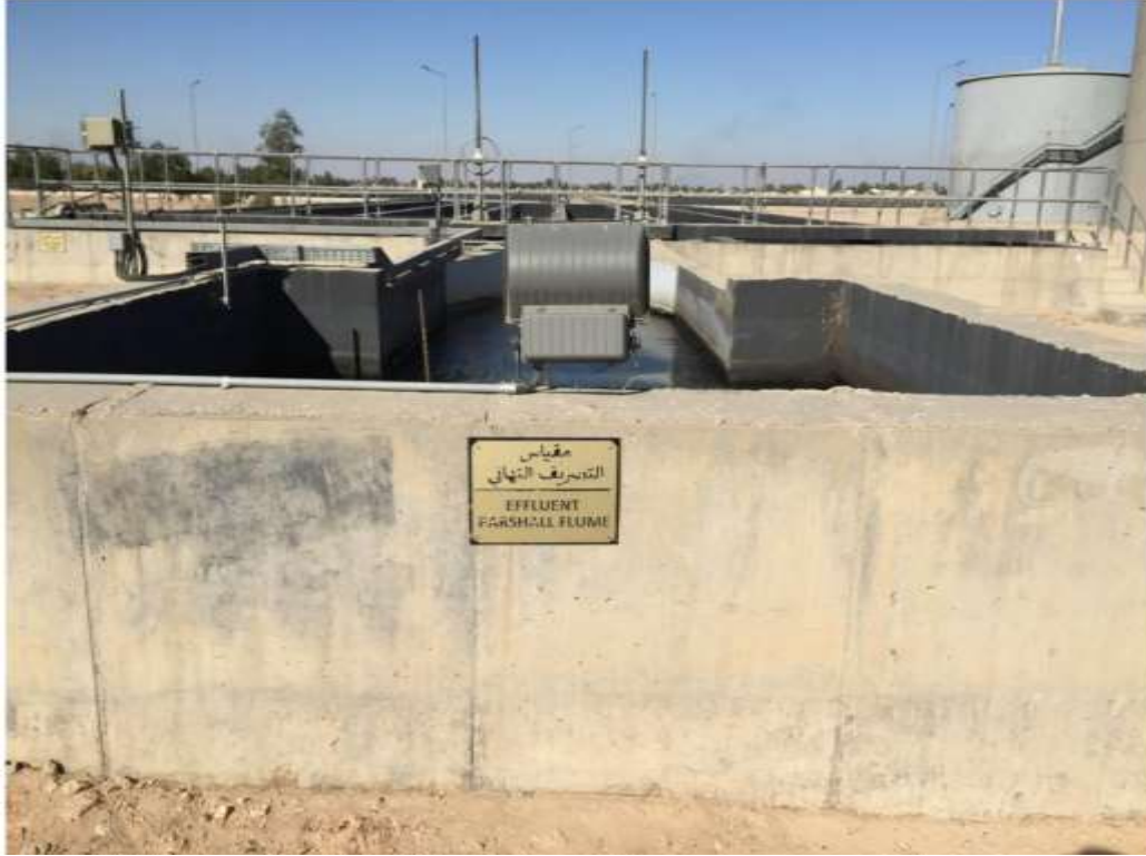
Figure 3-4: Parshall Flume Unit in Karbala WWTP.
