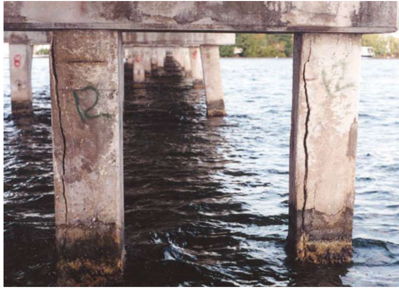
Figure 2-1. Corrosion in columns in marine structure (Moser et al., 2011).
