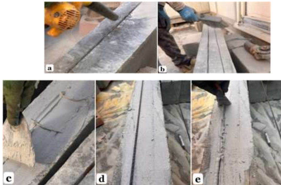
Plate 3-15: Stages of installation CFRP bar and CFRP strip, (a) Clean the grooves by air pressure, (b) Clean the grooves by brush, (c) grooves were filled with the epoxy, (d) Insert the bar into the grooves, (e) Surface leveling.
