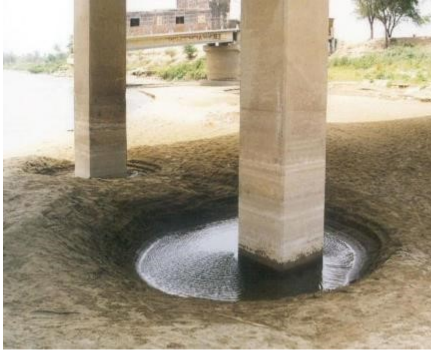
Figure 2-3: Photo of local scour around rectangular piers (www.pepevasquez.com).
