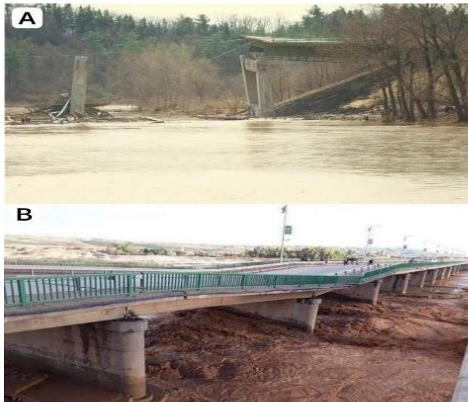
Figure 1-1: Bridge failure cases (A) Schoharie Creek Bridge (National Transportation Safety Board (NTSB), 1987), (B) Daquq Bridge (www.nrttv.com).
